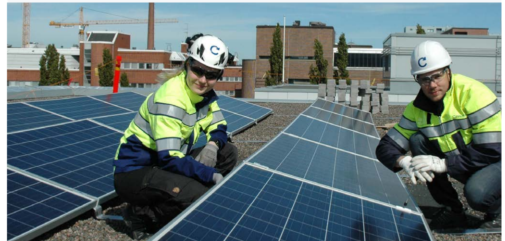
Project Manager Rea Tiehaara and Maintenance Manager Jussi Wacklin from Caverion inspected the solar panels installed in summer 2016.
